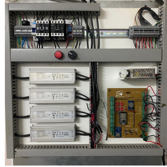
(b) Electronics panel with ESP32 and control modules.
